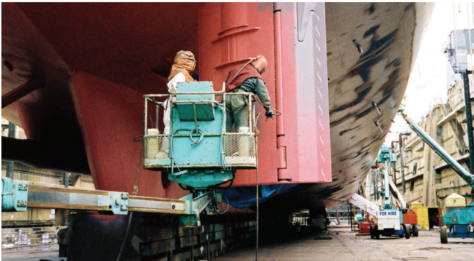
Coating application in a dry dock situation is often done with considerable time constraints. Equipment reliability is crucial.
