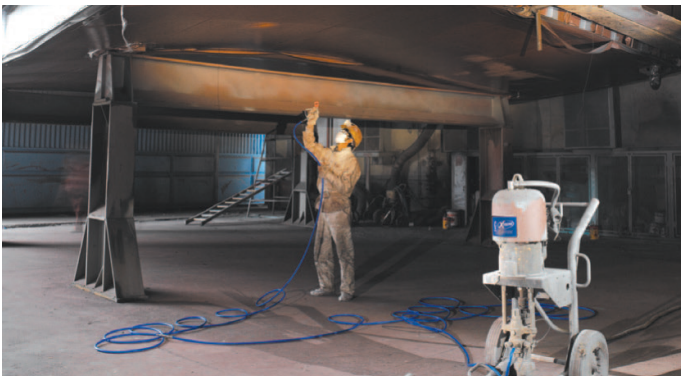
Coating application of a ship's module is simplified in a dedicated painting and drying room. Temperature and humidity can be constantly maintained 365 days a year.
